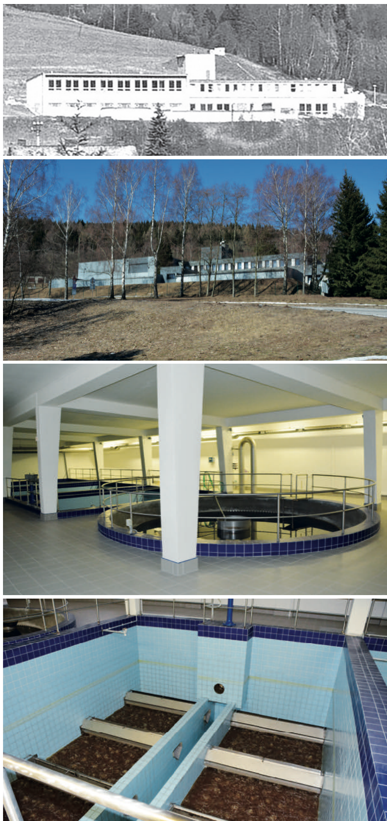
Fig. 5. Water treatment plant at the time of construction (ŠPVS archive), after reconstruction in 2008, the filters hall with reaction tank and filters, filter scrubbing (March 2022, A. Létal)
