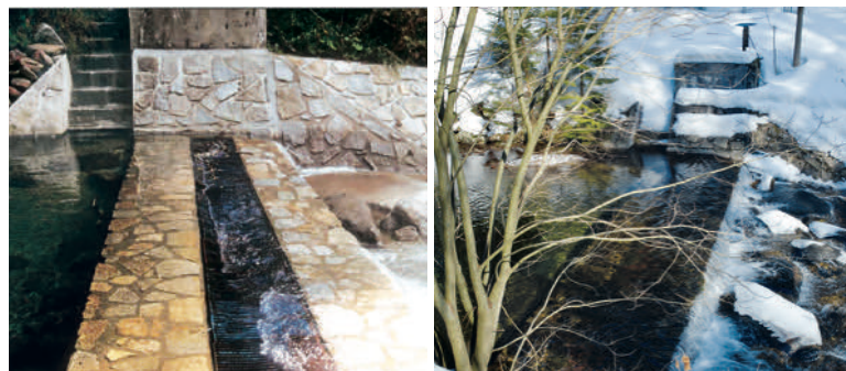
Fig. 10. Intake structure on Hučivá Desná river, state after construction in 1997 (ŠPVS archive), current state on the right (March 2022, A. Létal)
