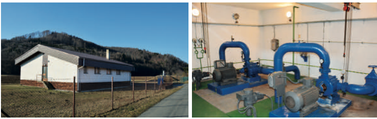
Fig. 7. Rapotín Water Treatment Plant with intake well (left), engine room (right) (March 2022, A. Létal)
